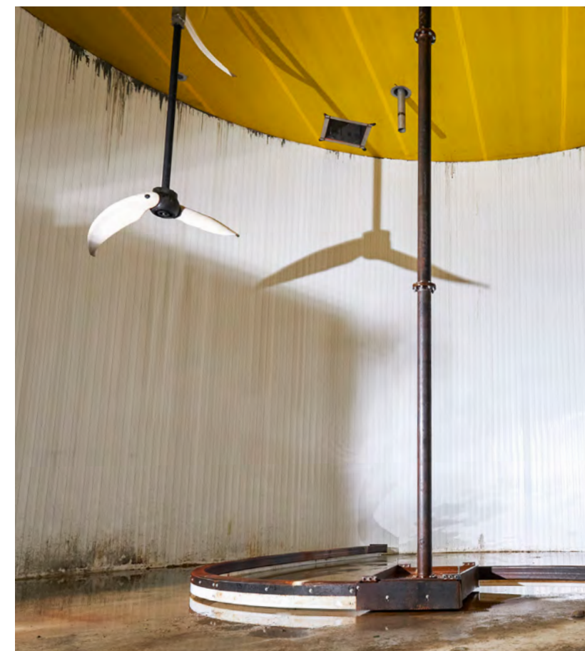
Agitator and Floor Sweeper inside ZooShare's Self-Cleaning Digester
