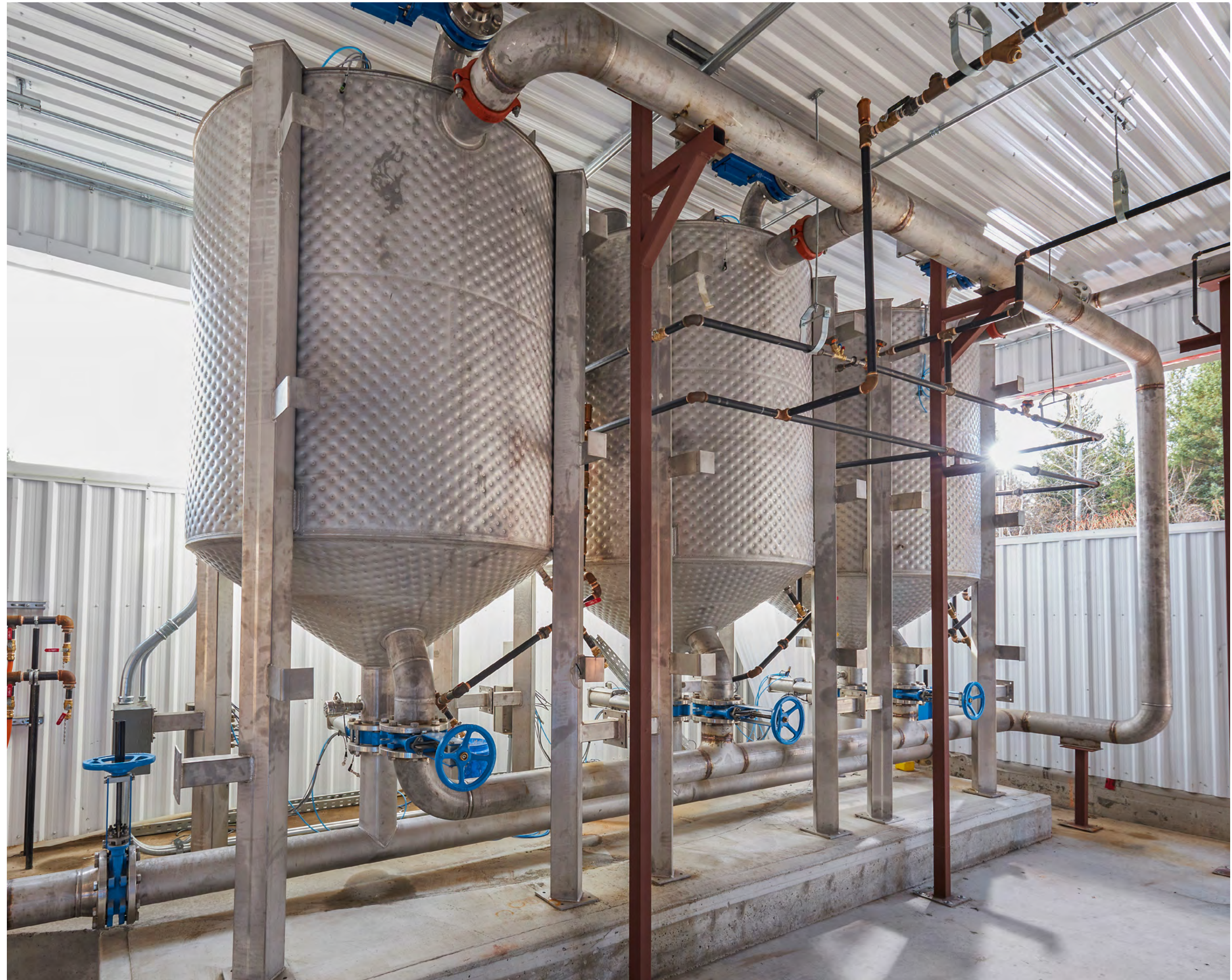
Holding tanks at ZooShare biogas plant in Toronto, Ontario
