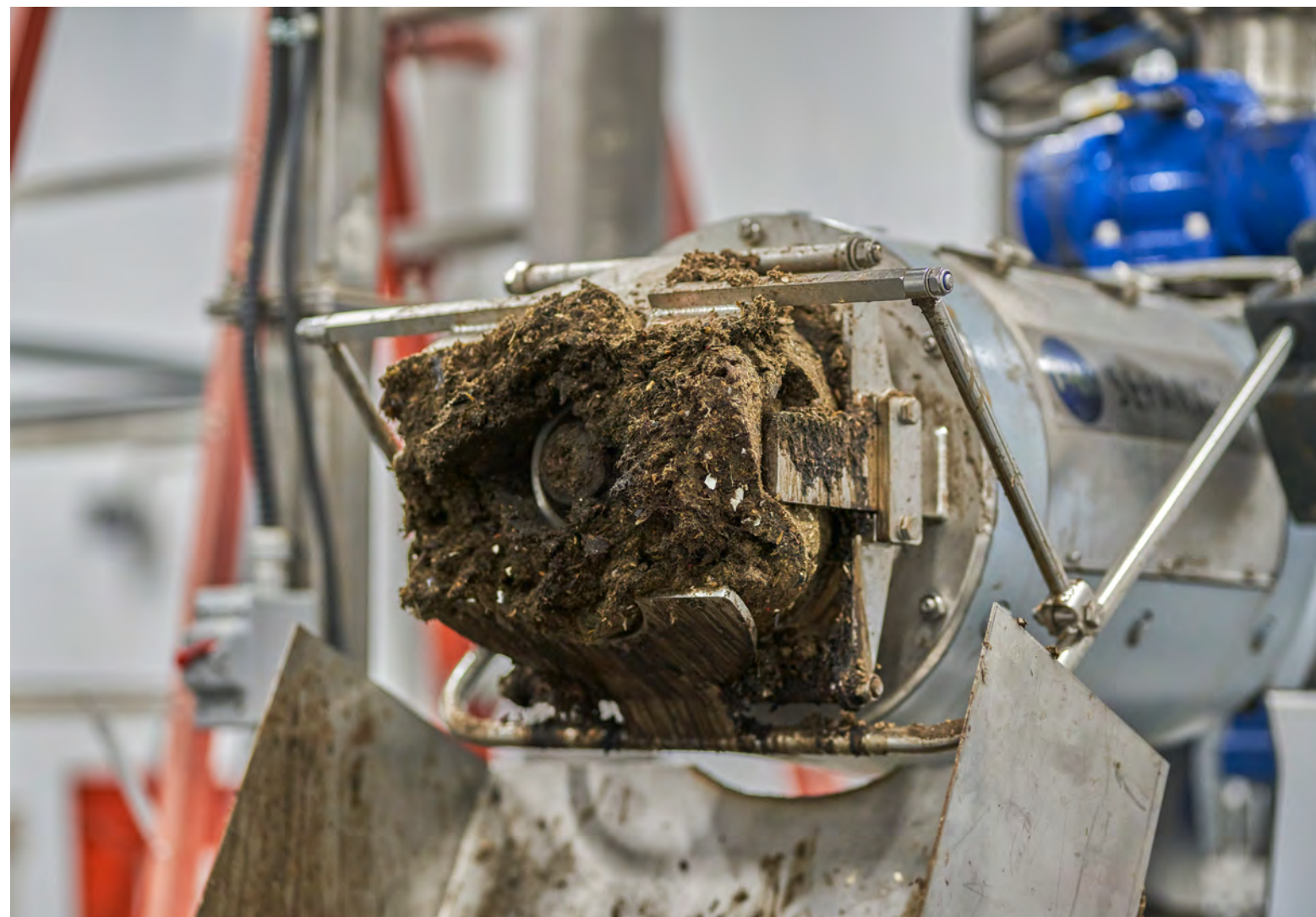
Screw Press squeezing out floating contaminants
